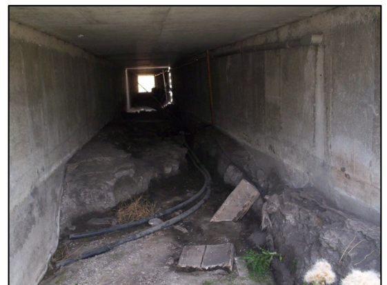
Debris and sediment inside the stock pass culvert at MP 157.2
